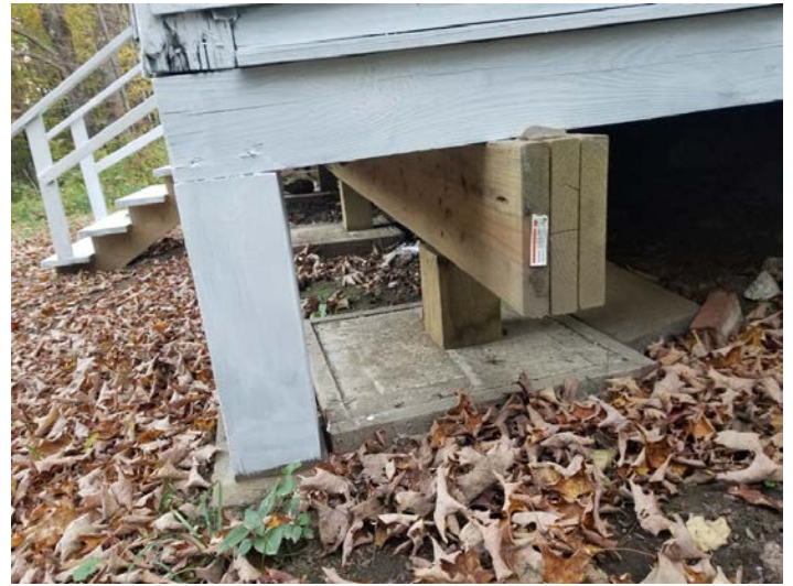
And a beam was added as required by the Insurance!
