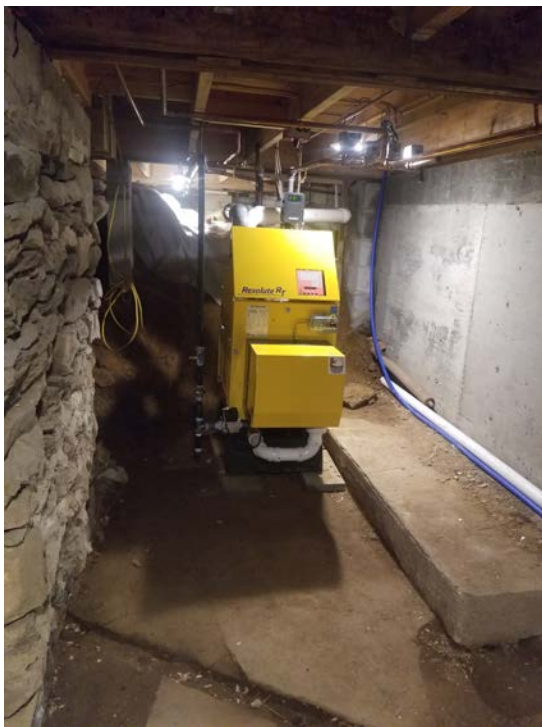
The new furnace, installed with support from a Vermont Cultural Facilities Grant
