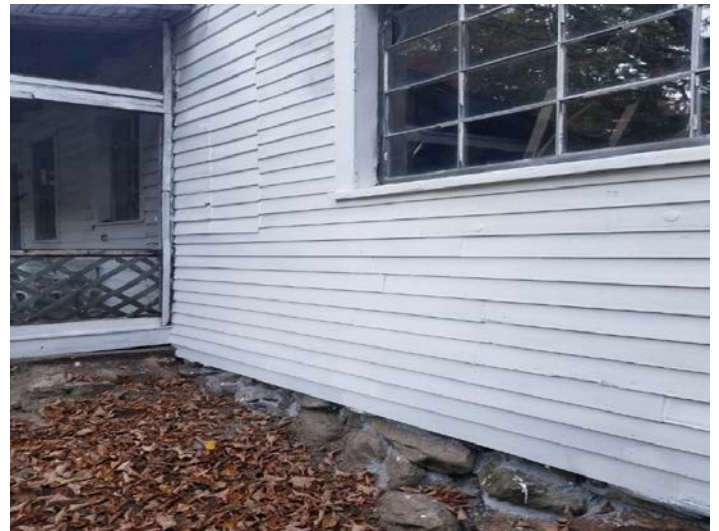
This is the same spot...the beam replaced and the missing siding put back on! This work required guidance from a structural engineer!
