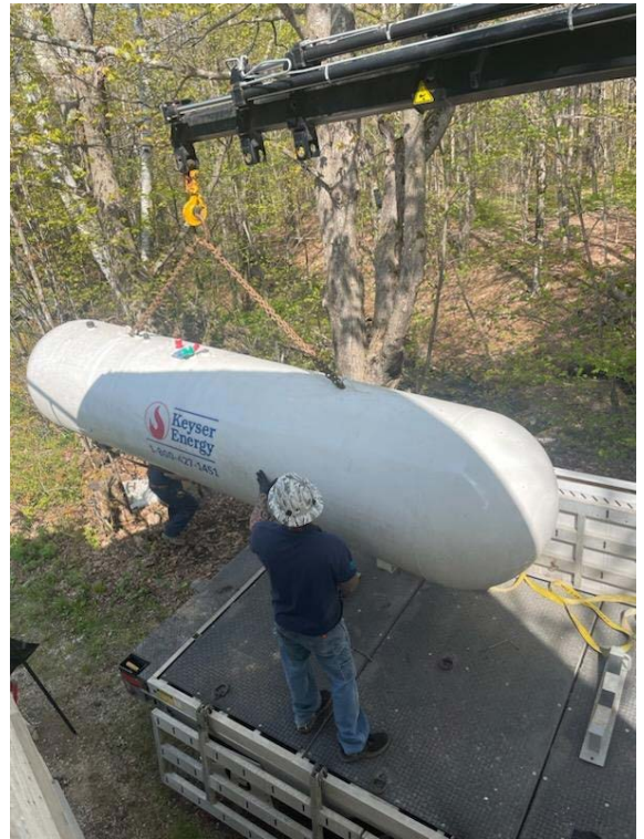
Setting of the 1000 gallon propane tank, sized for both heating the house and a backup generator yet to be installed
