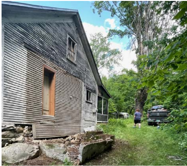
Before photo, broken windows, unpainted, foundation from shed still hanging on
