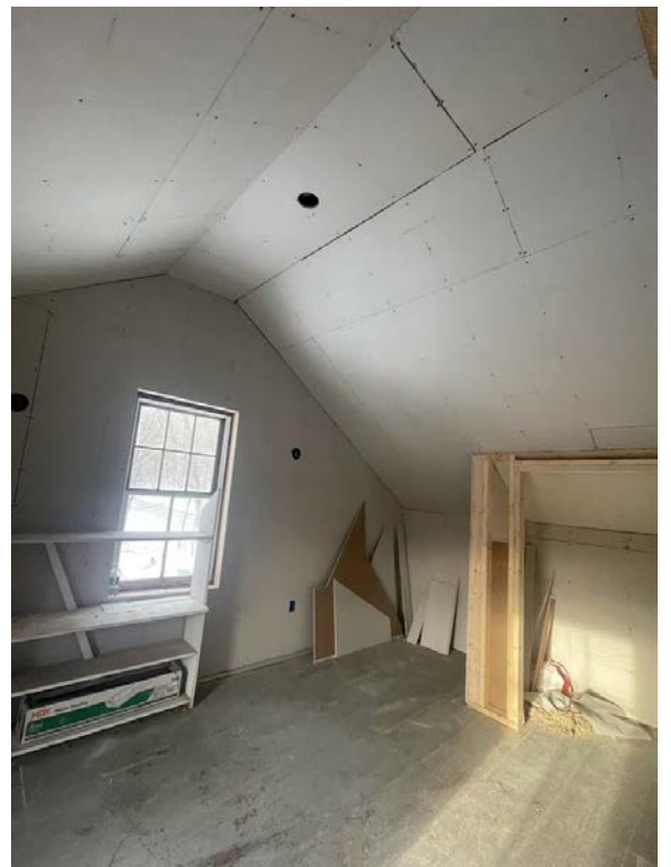
All new electrical and drywall also installed and new fixtures in the upstairs bathroom.
