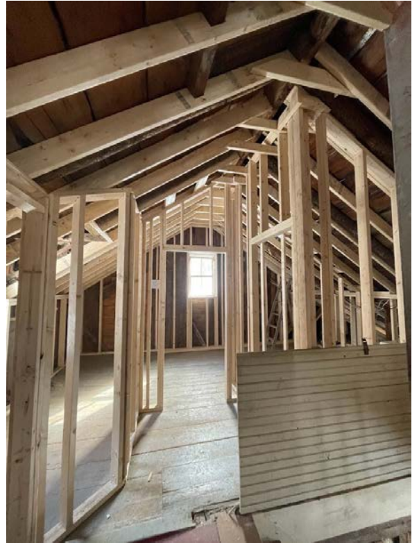
It was then reframed with additional vaulted rafters that added some necessary support as many of the original rafters were failing (or had already failed).
