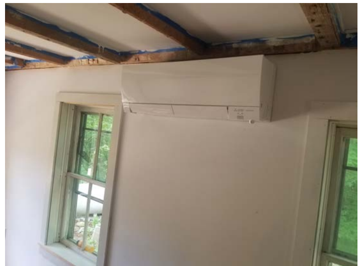
One of two heat pumps, this one a multi-split, installed at the same time.
