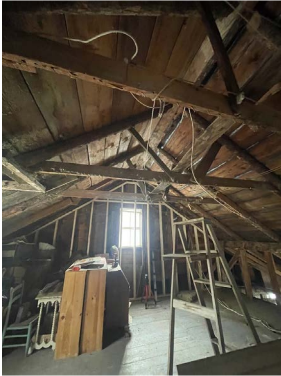
The second floor was torn down to the studs as they like to say.
