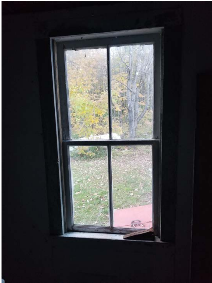
Original window with lead paint
