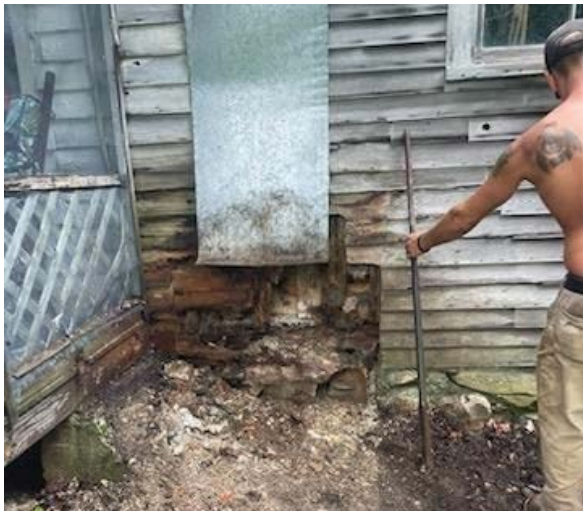
There used to be a chimney here, it was half removed and the beam behind it had rotted away
