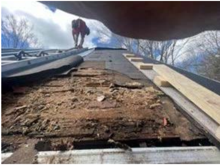
Repairs to the upstairs made it apparent that the roof on the side of the house with dormers needed to be replaced, and the dormers were flashed so poorly that a large chunk of beam needed to be replaced as well.
