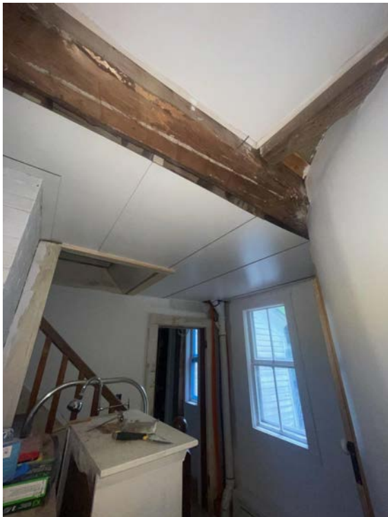
The ceiling around the fireplace on the fire floor was also installed, the back wall finished by the stairs, and a new sewage pipe installed in a less obvious place. Other minor finishing work was also completed on the first floor.
